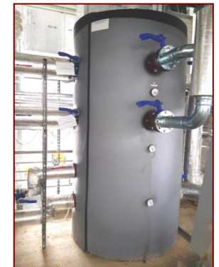
View of the 3 m 3 buffer tank
