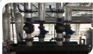
Waste heat distributor
