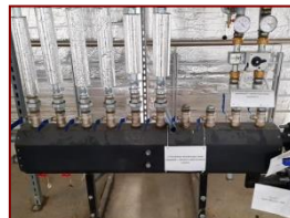
Manifold distributing heat to social islands
